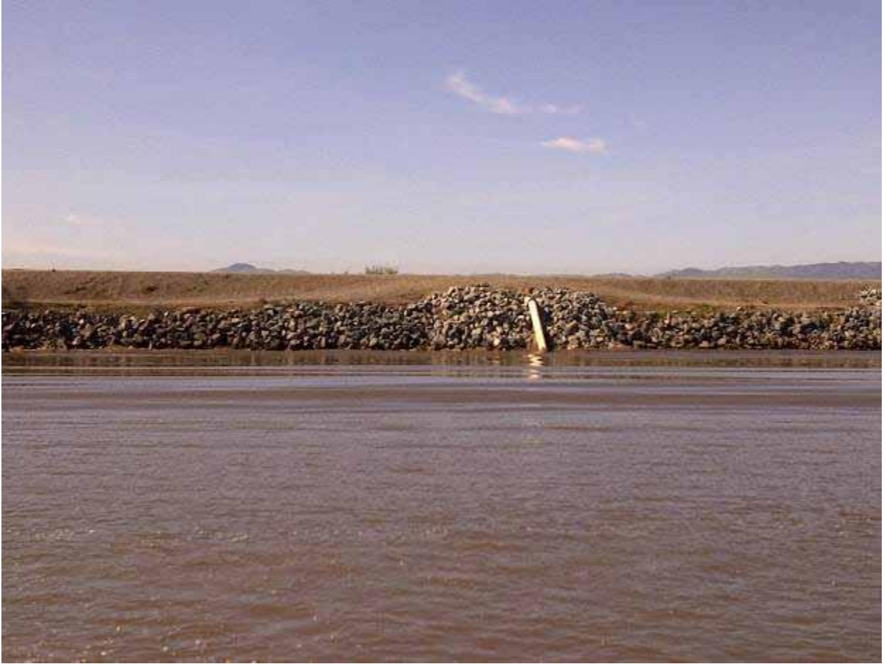
Figure C-8 - Byron Tract, showing stepped seismically-resistant levee
